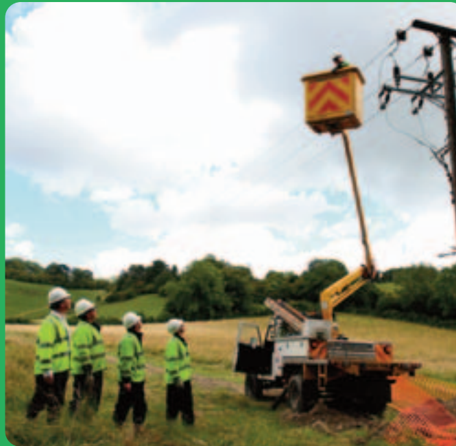
Overhead equipment is deactivated and installed underground to make beautiful landscapes even more spectacular
