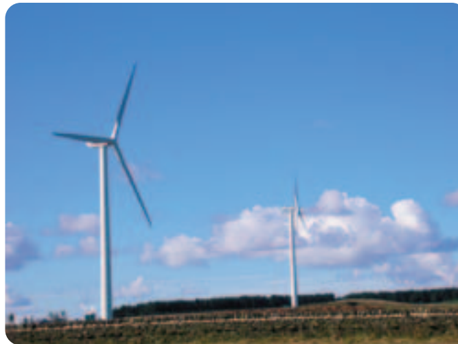
Windfarms are part of the sustainable projects developed by EDF Energy
