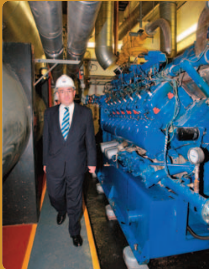
Energy minister Malcom Wicks visits our CHP station at Barkantine
