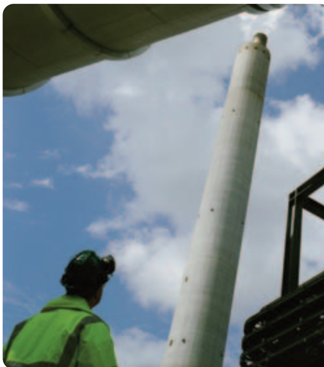
Sutton Bridge Power station
