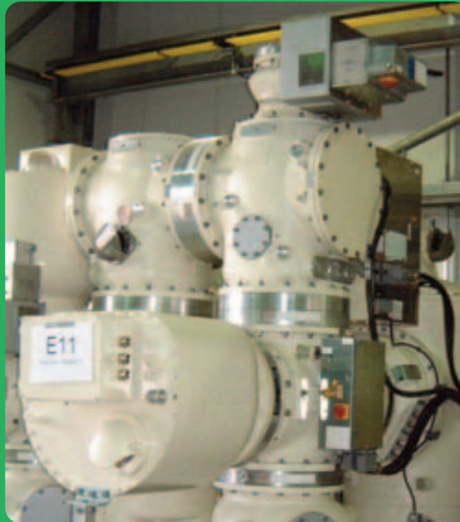
132kV substation: SF6 filled equipment
