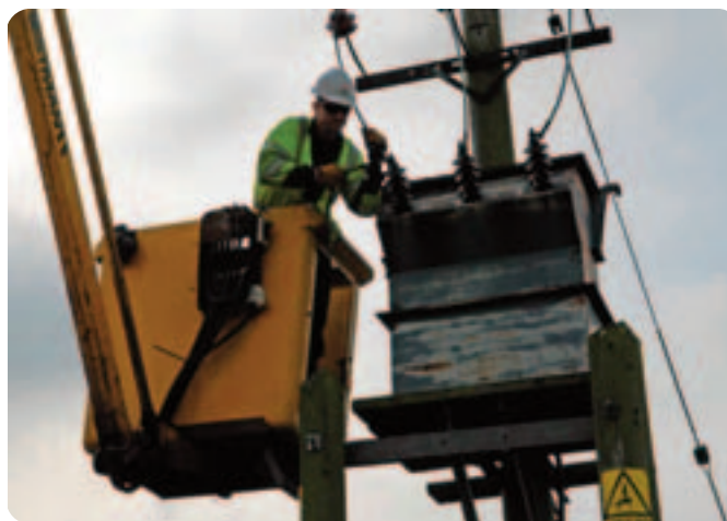
Investing in the network to ensure continuity of supply
